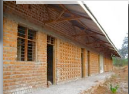
New Clinic and Dispensary at Ibambo. This very large clinic will eventually act as a district health centre.
