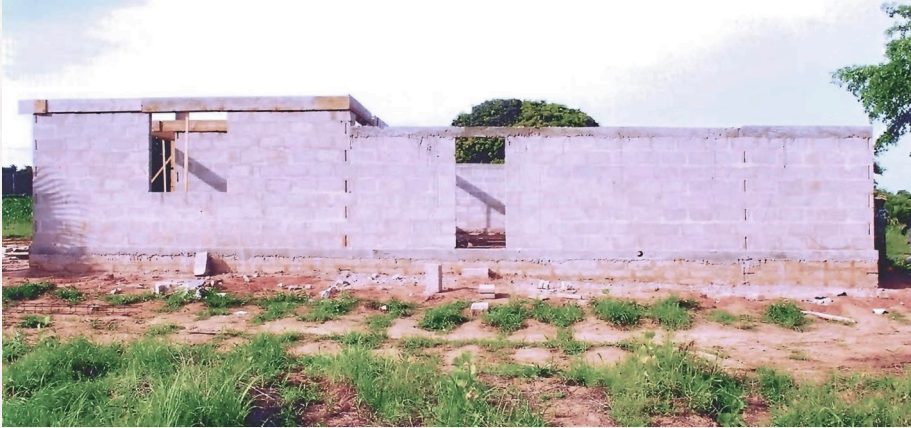
The Mwanhala Clinic staff house is up to the level of the lintels
